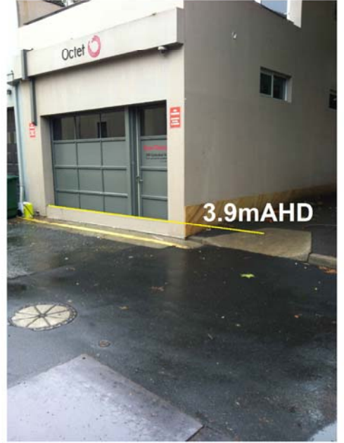
Flood barrier installed at Bossley Terrace, with approximate elevation of barrier height. 3.9m AHD
