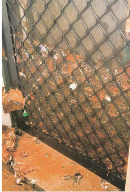
Floodmarks at residence entrance on Victoria St.
