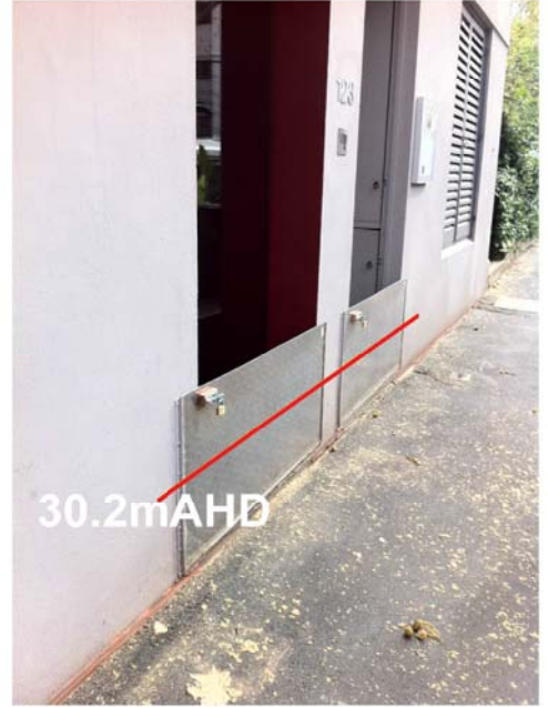
Floodgates installed to avoid inundation at Victoria St, with approximate elevation of flooding in February 2010.
